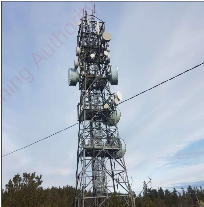
Figure 9.5. Shanettra - Mast A1
